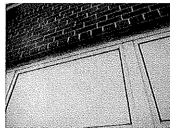
Photo 10 Rust at lintel of 1950s addition.
