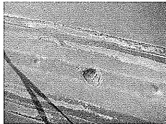
Photo 16 Raised fastener penetrating the roofing membrane with failed sealant repair.
