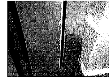
Photo 12 Failed window perimeter sealant.
