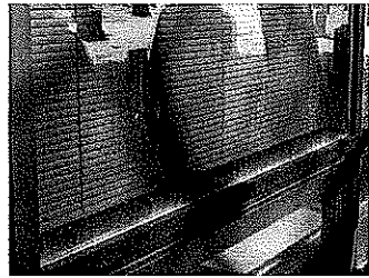
Photo 23 Faded IGU along east elevation curtain wall.
