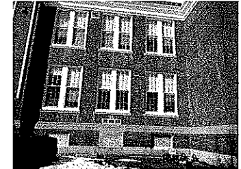
Photo 4 Grey staining below windows at south elevation of 1927 Building.
