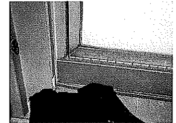
Photo 20 Falling window glazing.
