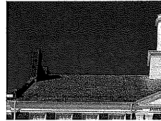
Photo 18 Patched areas in slate roof.
