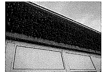
Photo 11 Cracks in band course elements above rusted lintel.
