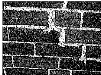
Photo 7 Failed mortar repairs at chimney.
