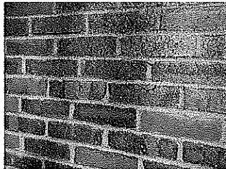
Photo 16 Cracked and variable-colored brick typical at 1979 Addition.
