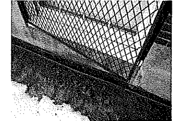
Photo 4 Rusted and broken window grates.
