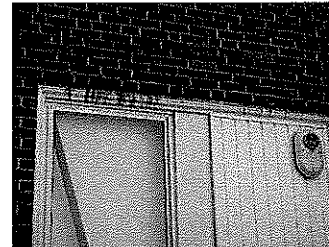
Photo 2 Corrosion of lintel and localized mortar joint repairs at 1927 Building.
