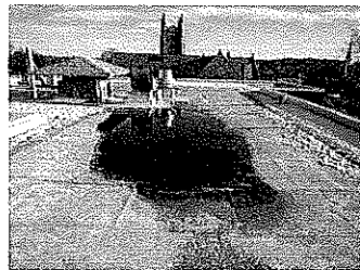
Photo 16 Ponding water at roof.
