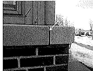
Photo 9 Open joints in precast concrete sill at northeast building corner (yellow arrow). Open joints in window framing and crazing/debonded perimeter seals (red arrows).
