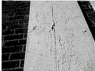
Photo 7 Peeling paint at decorative wood elements of 1927 Building.
