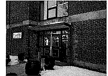
Photo 3 Staining, efflorescence, and organic growth on brick masonry below canopy.
