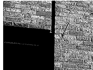
Photo 17 Step cracking in brick masonry at end of auto shop garage door.
