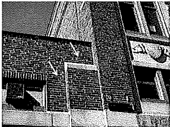
Photo 14 Slap crack emanating from upper right window corner of one-story 1950s addition.
