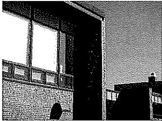
Photo 5 Efflorescence and spalling brick at old East Junior School, south elevation, wing wall.
