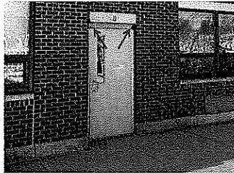
Photo 15 Corrosion at hollow metal door frame.
