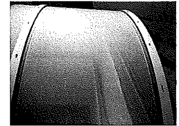
Photo 27 Micro-cracking of skylight acrylic glazing.
