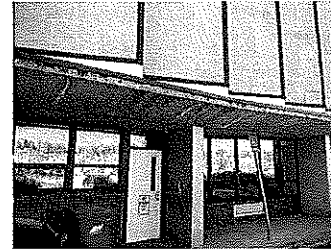
Photo 9 Cracks and efflorescence in old East Junior School cafeteria/auditorium canopy.
