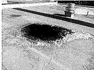
Photo 24 Ponding water on roofing membrane.
