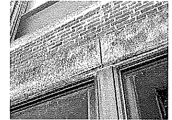
Photo 4 Corroded lintel with displaced precast band course above.
