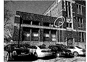
Photo 12 Efflorescence in brick masonry at one-story 1950s addition (red arrows). Yellow arrow points to location of step cracking in brick masonry; see Photo 14 for close-up.
