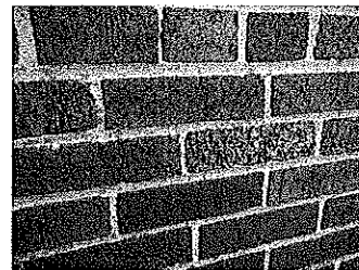
Photo 9 Condition of brick masonry at 1950s building where ivy has been removed.
