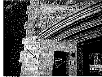
Photo 9 Dented and falling terra-cotta pieces at entrance.
