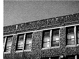
Photo 2 Efflorescence along outside of parapet at 1930 building.
