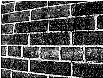
Photo 5 Deterioration of several bricks along west elevation.
