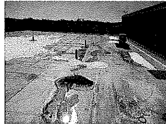
Photo 16 Ponding water at original Hosmer School Roof.
