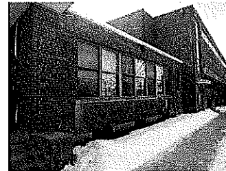
Photo 2 Efflorescence below window sill along north elevation.
