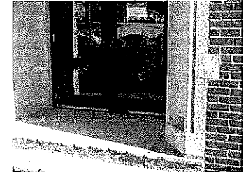
Photo 11 Broken and missing sweep at entrance door.
