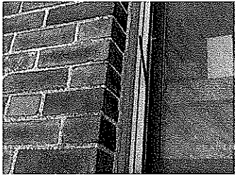
Photo 13 Cracked and falling perimeter seal at window.
