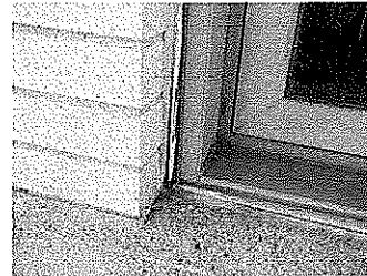
Photo 10 Close-up of perimeter sealant crazing and debonding at corner.
