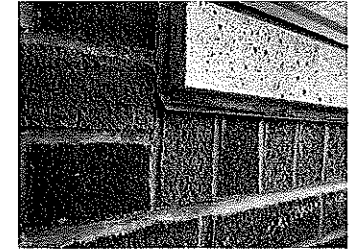
Photo 11 Typical condition at Connector Building. Metal flashing is flat-lapped. Masonry and mortar joints are in good condition.
