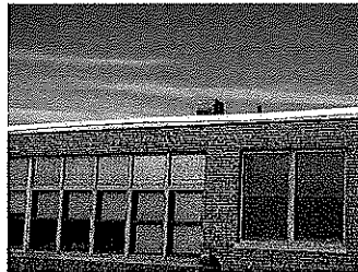
Photo 18 Displaced edge metal at 1954 Building roof.
