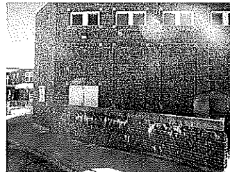
Photo 9 Efflorescence at site wall.
