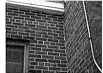
Photo 4 Step crack in brick masonry west of main entrance.
