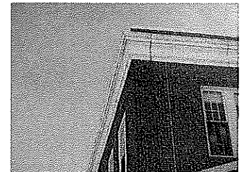
Photo 11 Metal cornice elements appear displaced at 1996 Addition.
