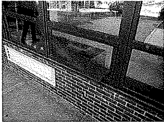
Photo 14 Broken screen at old East Junior School Cafeteria.
